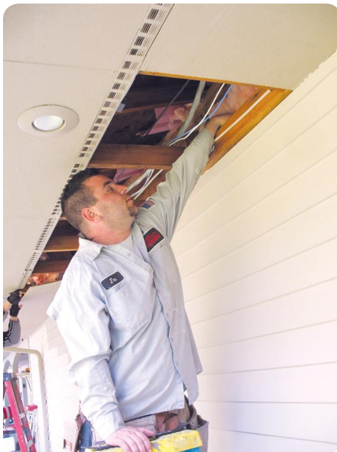
A GreenHomes America technician searches for the source of a pipe freezing in a bedroom wall.
