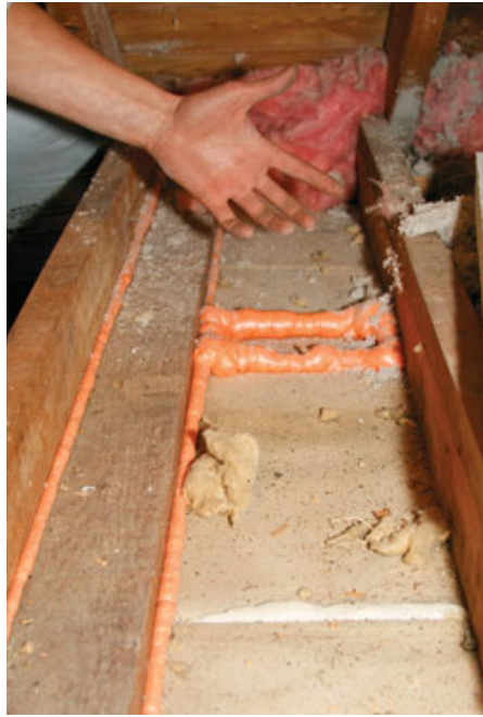
Figure 2. Crews seal spaces over cabinet soffits by installing rigid insulation across the opening at attic floor level and sealing the joints with foam (far left). Gaps where wall plates meet the attic floor must also be sealed (near left).
