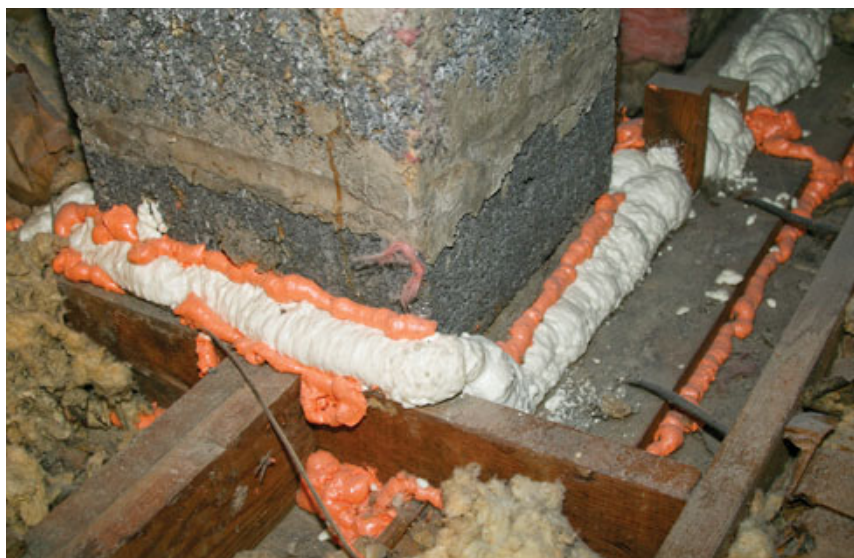
Figure 3. Can lights are covered with boxes made from duct board, which are foamed in place (top left); hvac boots are also sealed (top right). This chimney (above) was decommissioned when a direct-vent furnace was installed, so the crew has sealed around it with foam; air gaps around active chimneys are sealed using sheet metal and high-temperature silicone caulk.
