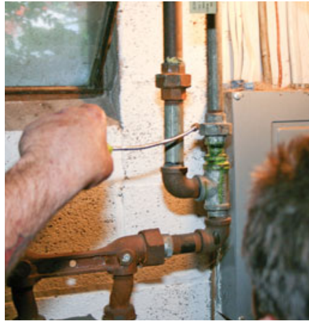
Figure 6. “Testing out” is a key element in quality assurance and customer service. In the house shown here, the technician saw the need to touch up the mastic on the basement ducts (far left). More important, he discovered a previously unnoticed gas leak (left) — a leak that probably became evident after other fittings in the piping were tightened.
