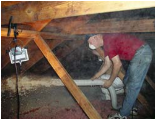
When blowing cellulose insulation into the attic, make it snug. "A few extra bags of insulation just doesn't add that much to the cost," says Tony Karpovich of GreenHomes America.
